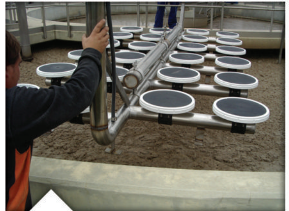
Disc diffusers provide exceptionally high oxygen transfer efficiency in this aeration tank in Spain.
