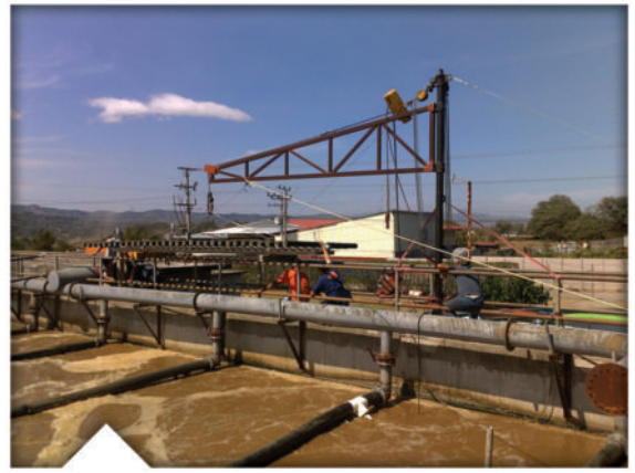
Retrievable grid with SSI Snappy Saddle™ Diffusers and a 304 SS frame replacing an underperforming floating lateral system
