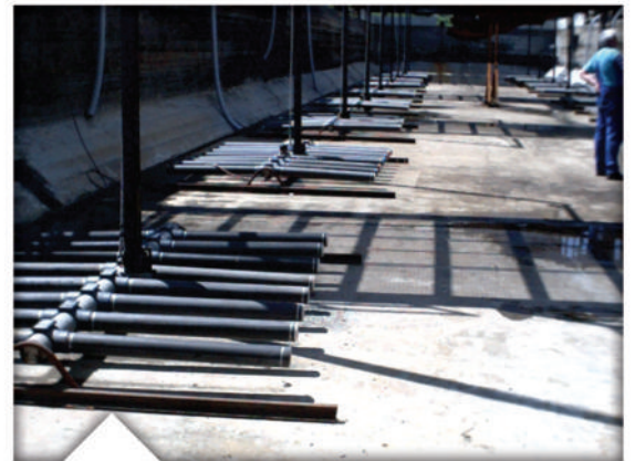
These liftable fine bubble tube grids on guide rails have worked over 10 years in this municipal WWTP
